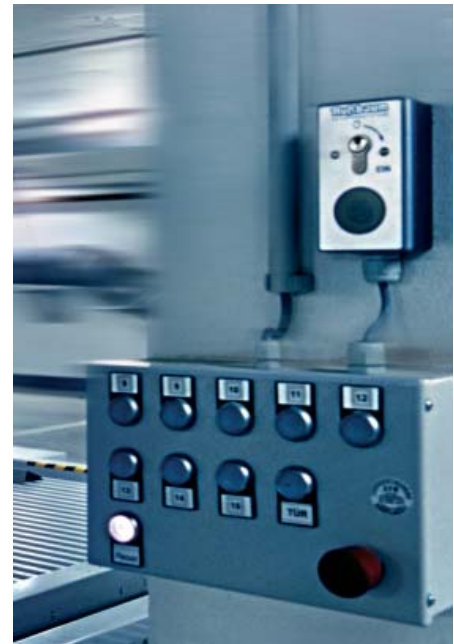
fig. above: operating panel with dead man's control (freely programmable execution)
